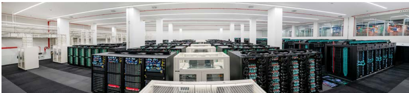
Located at Barcelona Supercomputing Center, MareNostrum 5 is one of the EuroHPC top-tier machines
