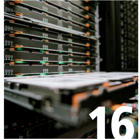
Data centres, storage and networking
